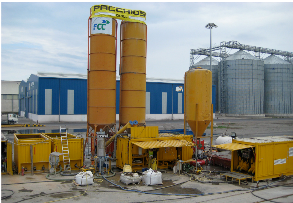
Fig. 4. General view of fixed installations
